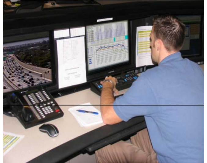
Express Lanes Operator monitors and manages 95 Express with CCTV and Express Lane Watcher application.
